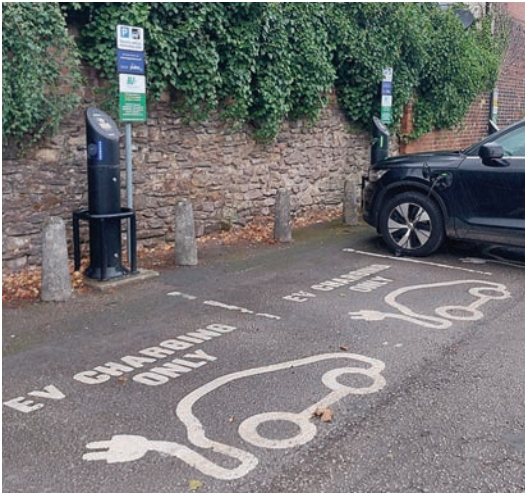
EV charging points at Field Lane Car Park, Belper
